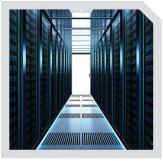
Data Center Cooling
